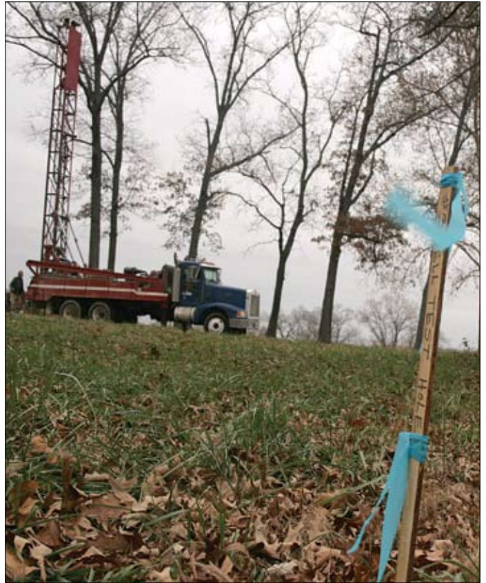
Pre-construction work began in December with test well drilling for the geothermal HVAC system.
